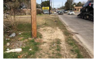
Sidewalks non-existent along major sections of project
