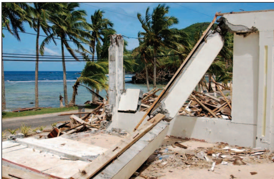
Figure 3-12. Damage from the 2009 tsunami (Amanave, American Samoa)
