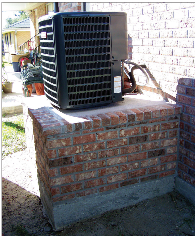
Figure 3-1. Air conditioning compressor elevated on a pedestal.
